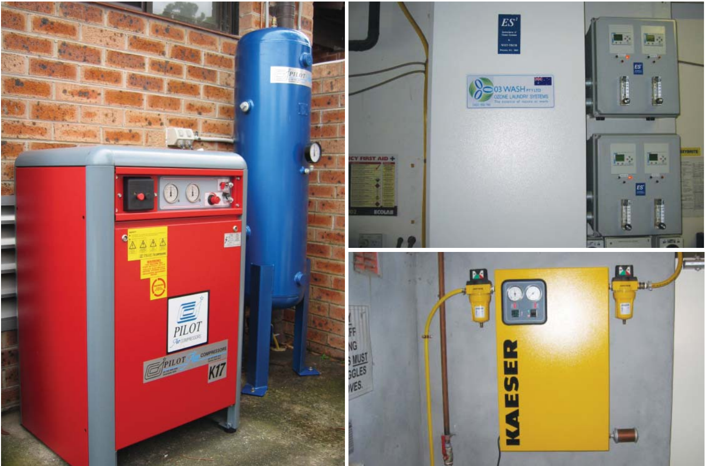
(Clockwise, from left) A 2 HP air compressor and a 20-gallon air storage tank used to pump air into the ozone system. Another ozone generating system. This one has the PLCs located to the right, rather than as part of a single unit. Another compressor that provides air for making ozone.
